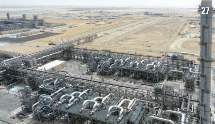
27. Manifa Gas Facilities Project Location: Khursaniyah, Saudi Arabia - Gas Inlet Facilities, Gas Processing: 90 MMSCFD - Condensate Stripping: 66,400 BPSD - SRU: 900 TPD×2 Project Period: 2008.08 ~ 2011.10
